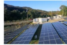
4.6 MW distributed solar power system with energy storage system in Ako, Japan
