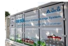
2MW/1MWh Energy Storage System for Xia Xing Power Station on Kinmen Island
