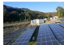
4.6 MW distributed solar power system with energy storage system in Ako, Japan
