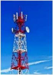
Outdoor telecom power solutions with integrated PV systems for a telecom operator in Africa
