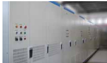
• Inverter to accompany in test
