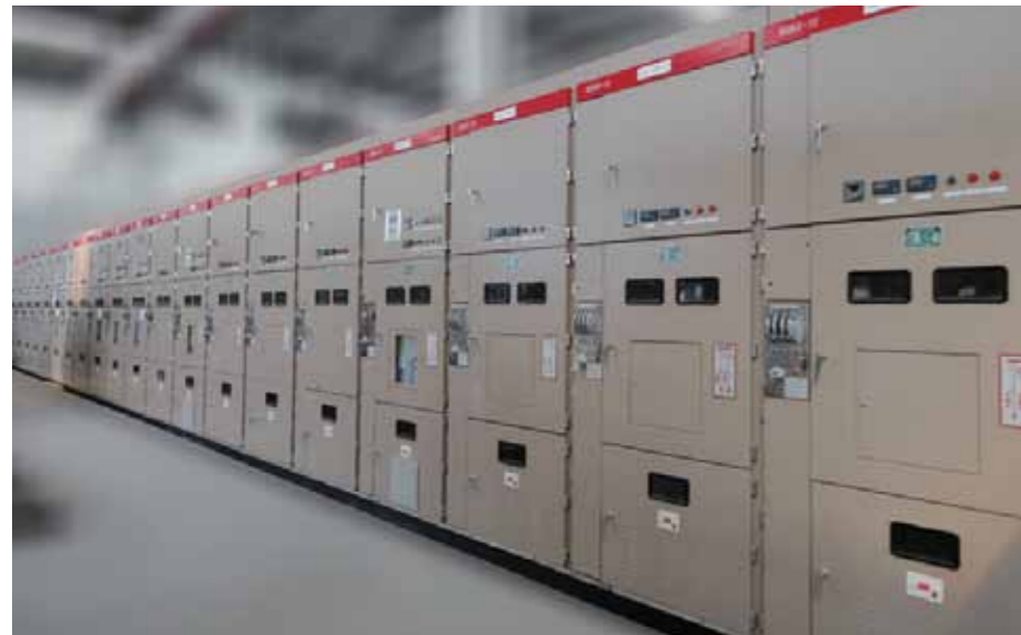
• High Voltage Distribution Cabinet System
