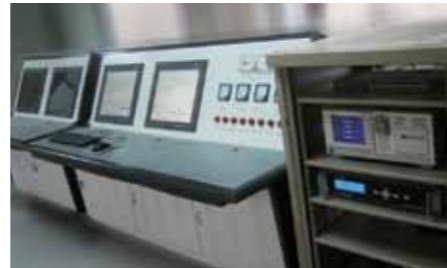
• Central control room
