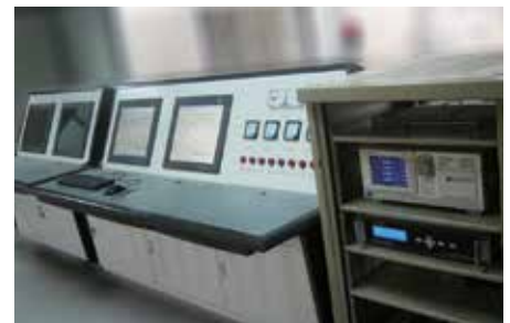
• Central Control Room
