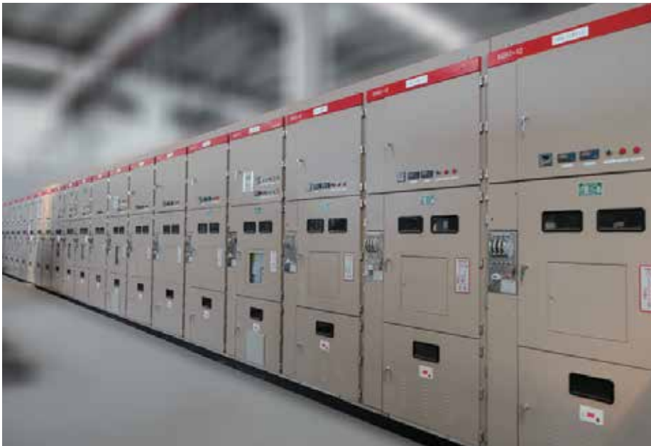
• High Voltage Distribution Cabinets
