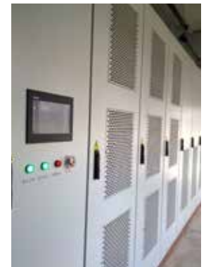
• MVD1000 for circulation water pump
