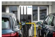
EV charging solutions installed all across Europe
