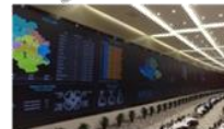
One of the world's largest video wall with 324 DLP 80" cubes and DVCS system in China
