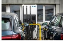
EV charging solutions installed all across Europe
